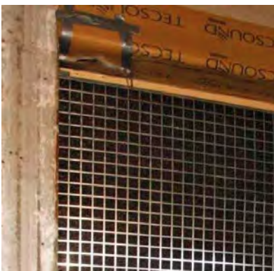
detail 4: detail on the top of the noise barrier. The opening was filled with a wooden beam and sealed with flexibel mastic tixotrophe
