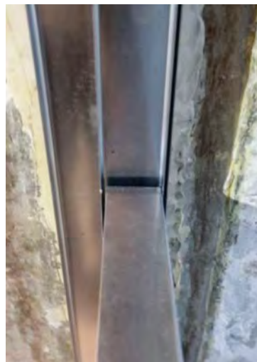
detail 2: U-profile on the side walls between the walls of the transmission room and panels
