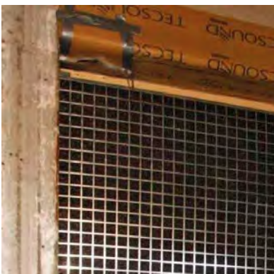
detail 4: detail on the top of the noise barrier. The opening was filled with a wooden beam and sealed with flexibel mastic tixotrophe
