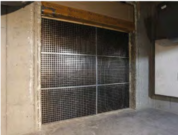
front side in the transmission room
