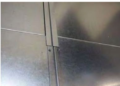
detail 1: I-profile at the location of the vertical joint between the 2 columns of noise barriers
