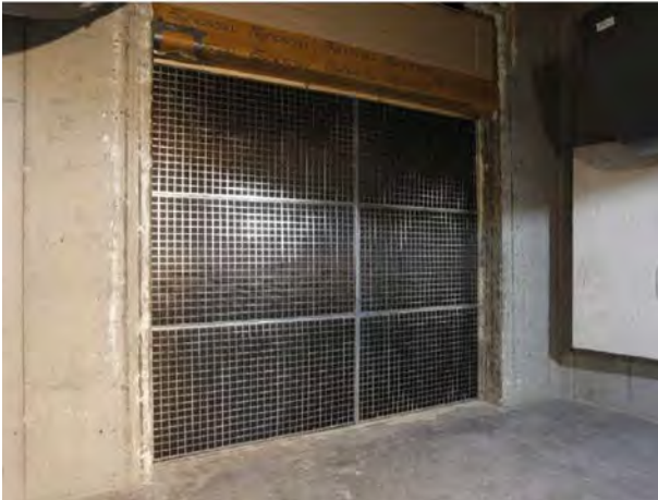
front side in the transmission room
